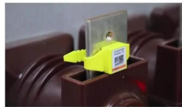
● Installed on Copper Busbar of Switchgear
